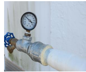
60 psi no leaks
